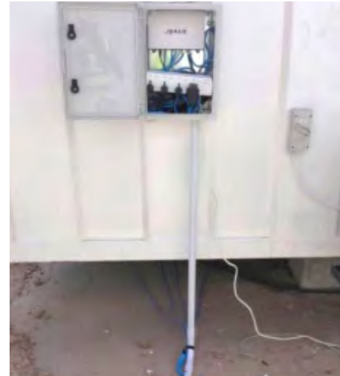
P2P links Neemrana Industrial Area | Rajasthan 2021
